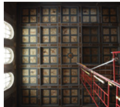
Top: ICA professional conservators at work on the ceiling of the Allen Memorial Art Museum at Oberlin College. Above: looking up at the ceiling.
